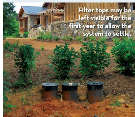
RAINWATER MANAGEMENT SOLUTIONS PHOTOS
